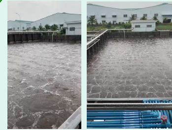
Evenly pool 調勻池
