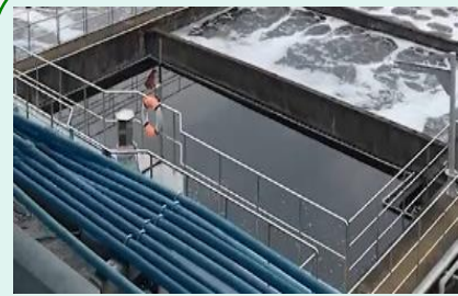
Final bio-precipitate pool 生物終沉池
